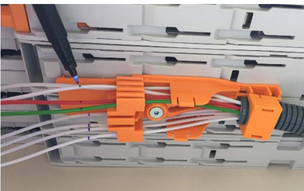
3.1.1 Mark the stripping point on the loose-tubes make sure that there is an overlap of 1cm behind the fopt-holder
